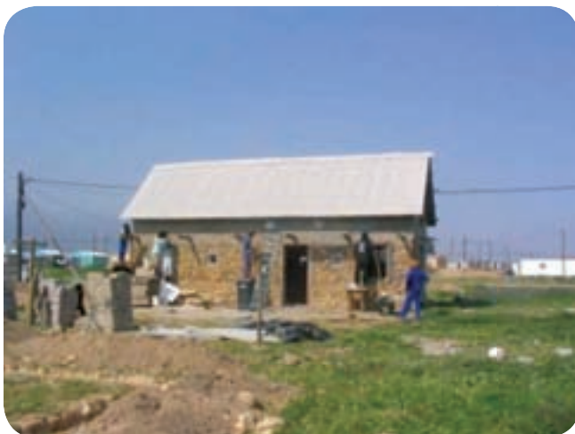
The 'Stonehouse' in Mbekweni under construction, with Cape Brick masonry in the foreground
